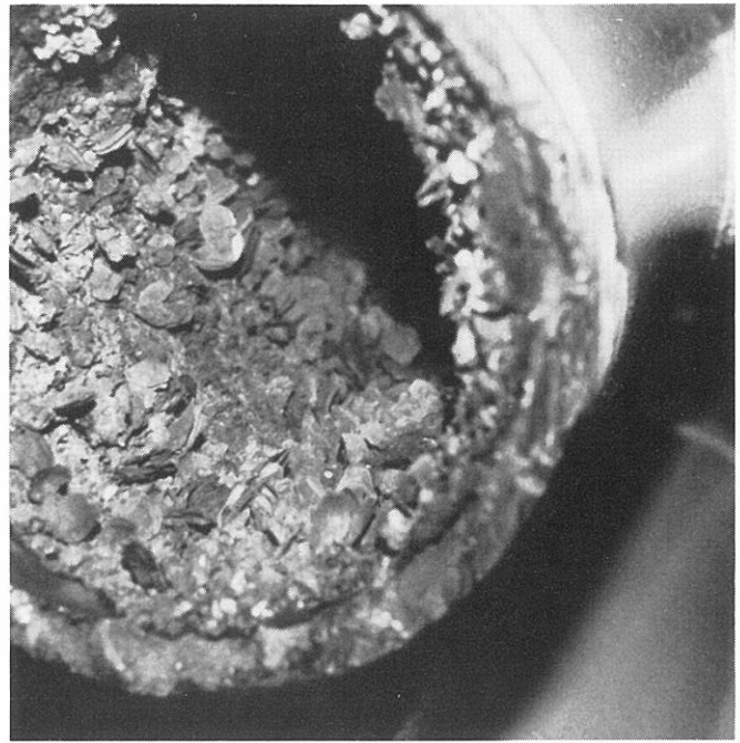
Fig. 1—Hard biofouling on an 8-in. Schedule 80 carbon steel header reduced the ID by 1⅞-in., and the cross-sectional area by 52% in just 2½ years of offshore service. Such fouling makes oversizing and frequent replacement of steel seawater piping components a practical necessity.
