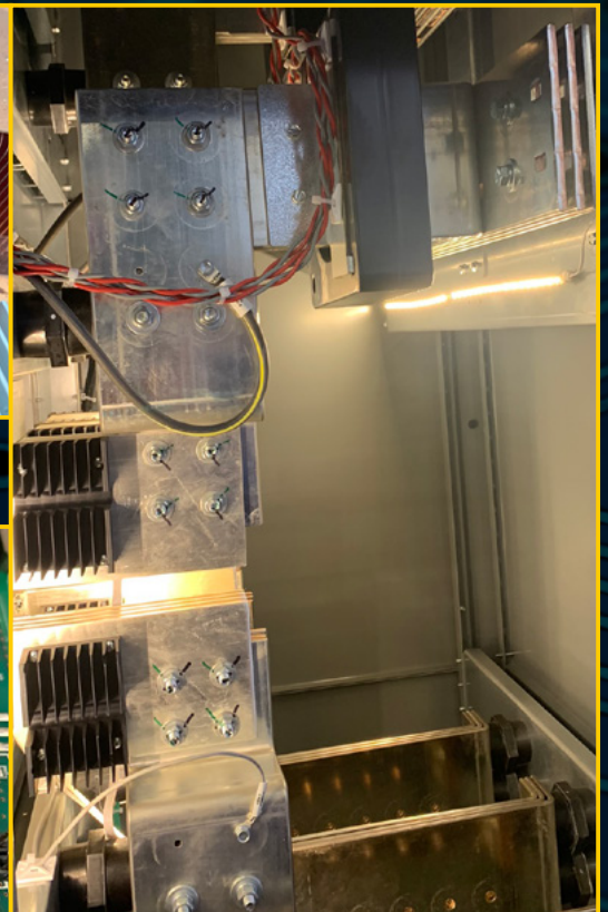
Figure 19: Plated Busbar conductors within Switchgear
