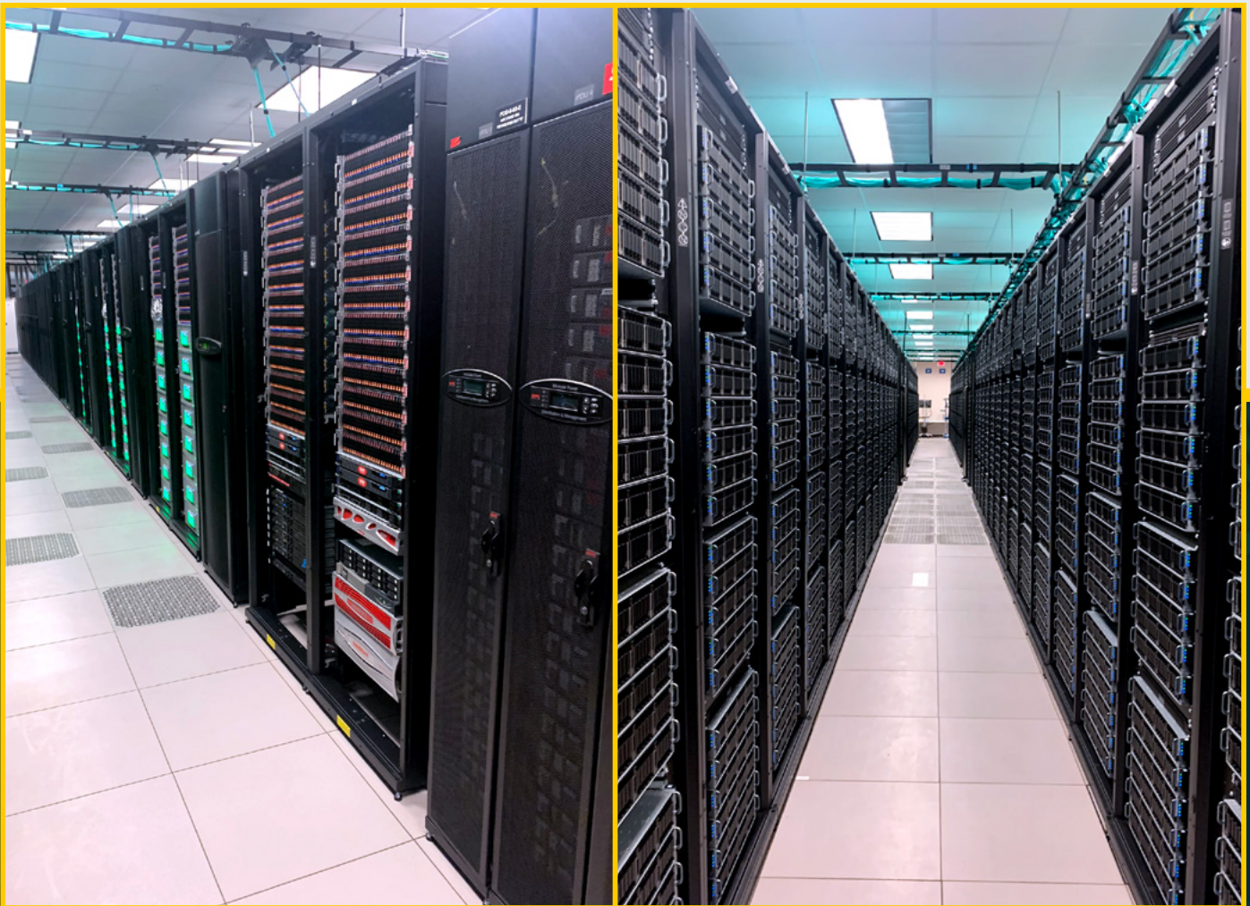
Figures 1 (left, cold aisle) and 2 (right, hot aisle): Racks of computing hardware in typical DCs
