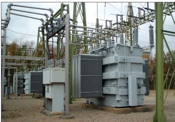
Figure 1. Much of Allegheny Power's distribution system is rural, with radial distribution. In order to ensure long life as well as low lifetime ownership costs, Allegheny Power insists that its power transformers be 100% wound in copper. Reliability is a key factor in transformers of this type.
